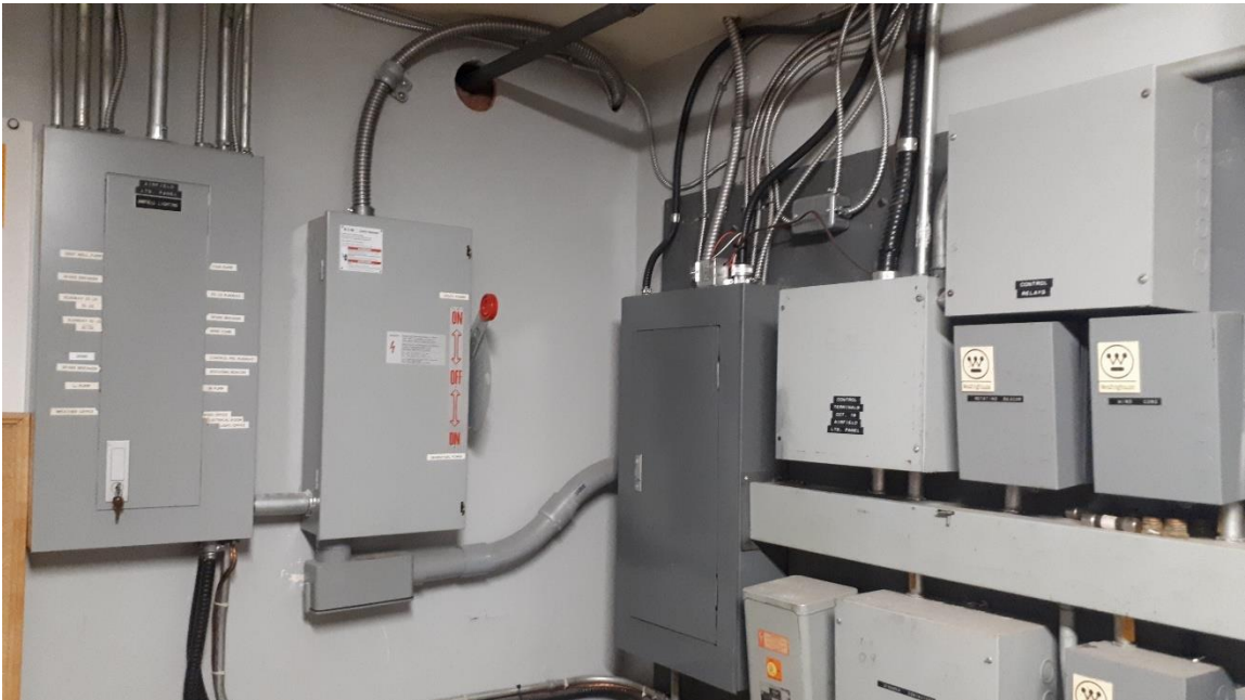
Terminal Building - Electric Panels
