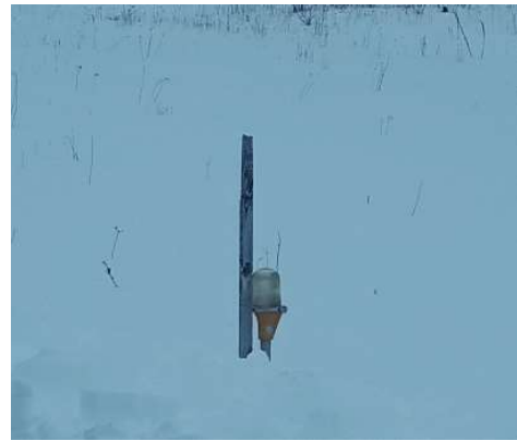
Figure 3-21 RWY 10-28 Edge Lights
