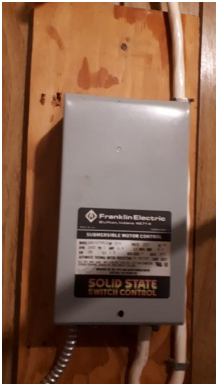
Terminal Building - Switch Control
