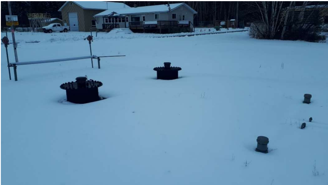
Figure 3-10 Air Fuel Underground Tanks
