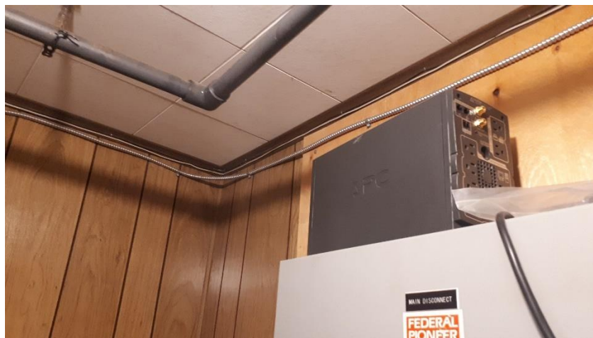
Terminal Building - Main Disconnect
