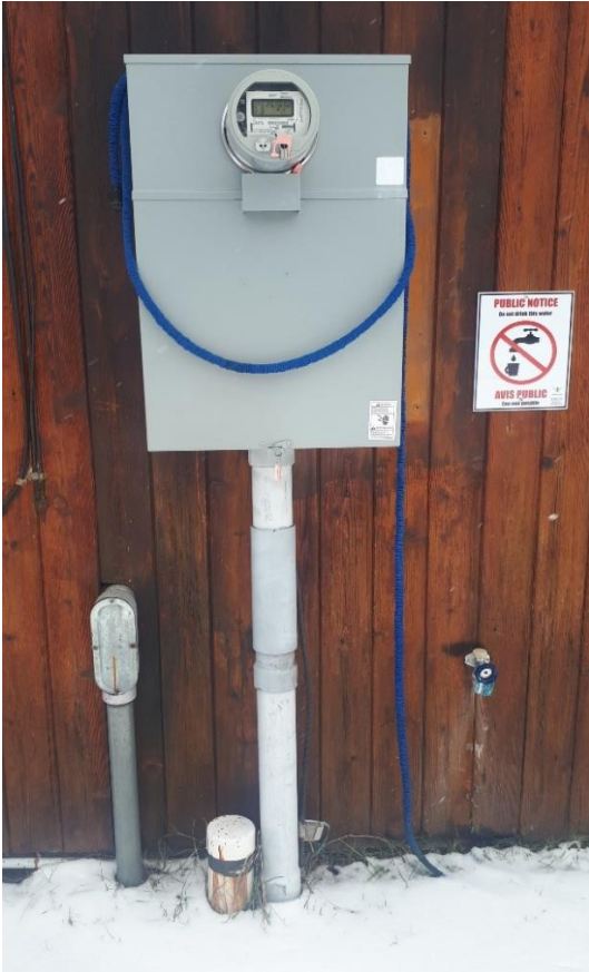
Terminal Building Hydro Meter
