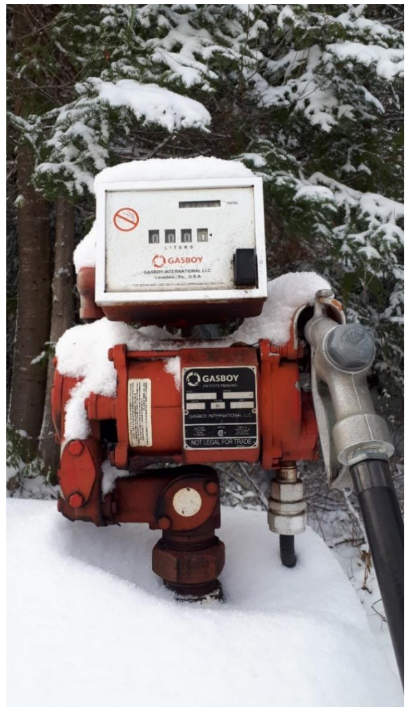
Fuel Dispenser and Meter/Gauge
