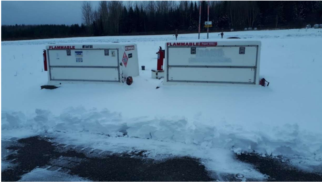
Figure 3-11 Jet and Aviation Gasoline Fuel Dispensers
