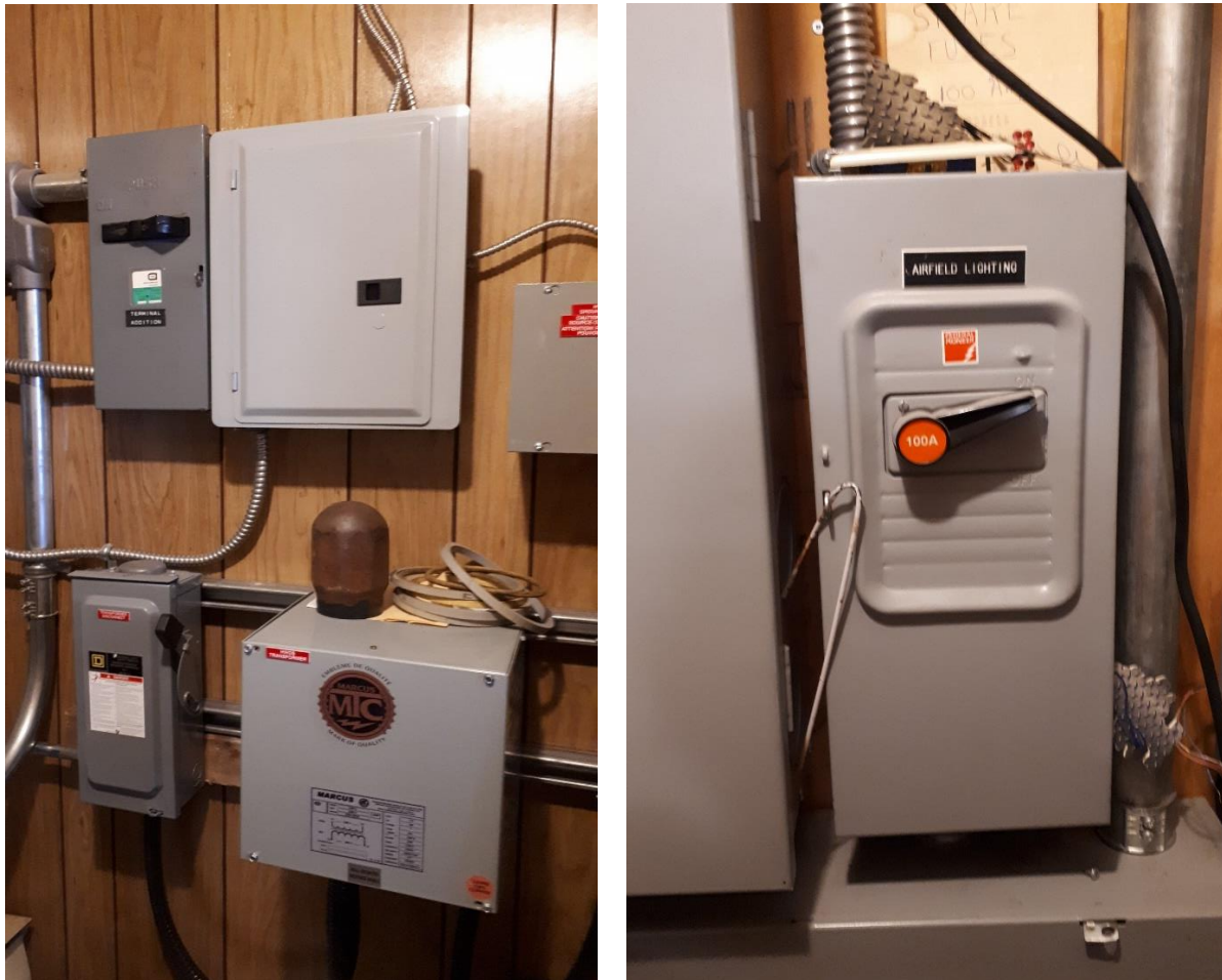
Terminal Building - Electric Panels, HWOS Transformer and Airfield Lighting Panel
