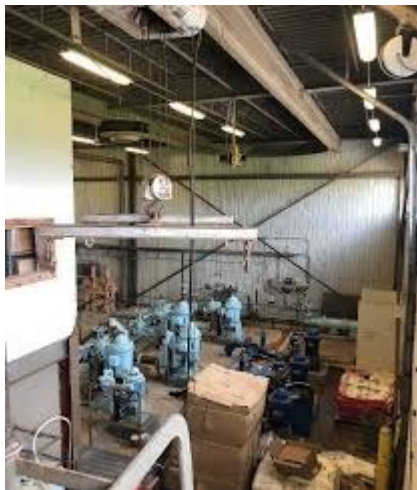
The Chapleau Water Treatment Plant is a critical asset for providing safe drinking water to the community. Image: Township of Chapleau
